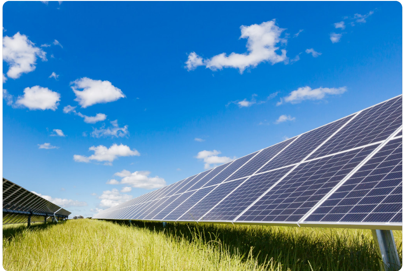
The solar panels Genesis will use at our first solar farm in Lauriston, Canterbury
