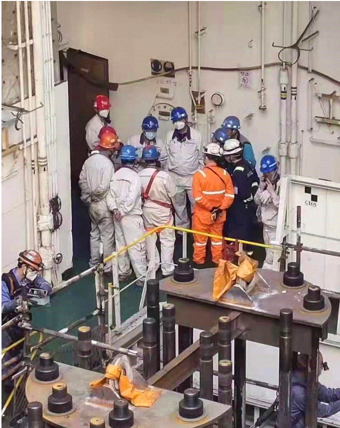
Workers at the China shipyard for the construction of the FPSO facility.
