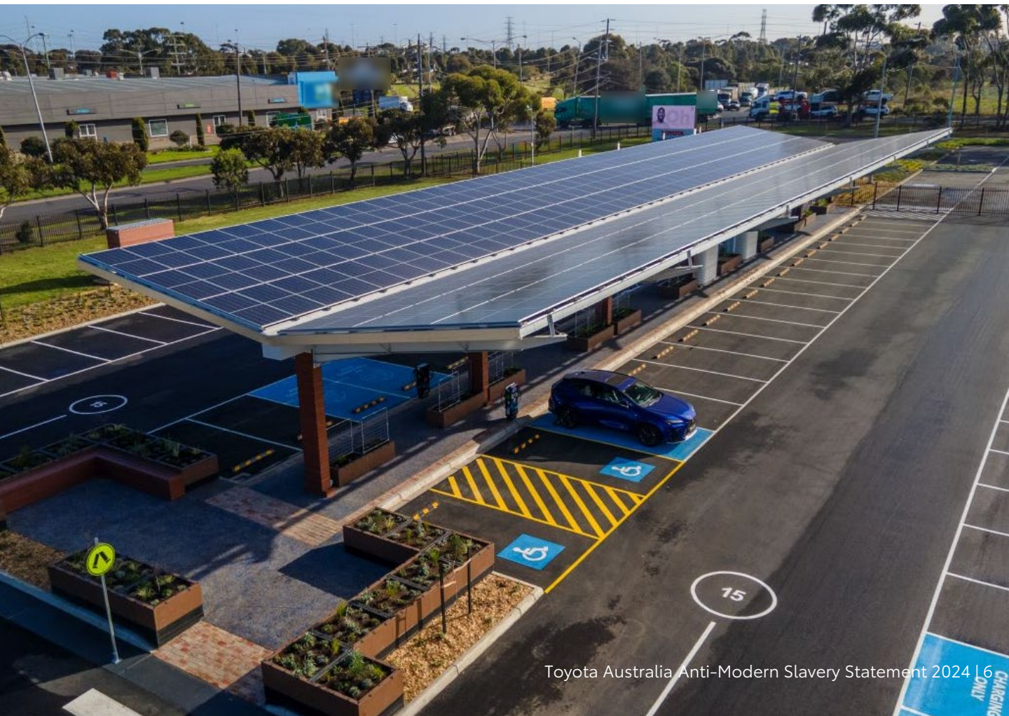
Solar Carpark at Toyota's Centre of Excellence in Altona North, Victoria. An example of due diligence and sustainable procurement practices.
