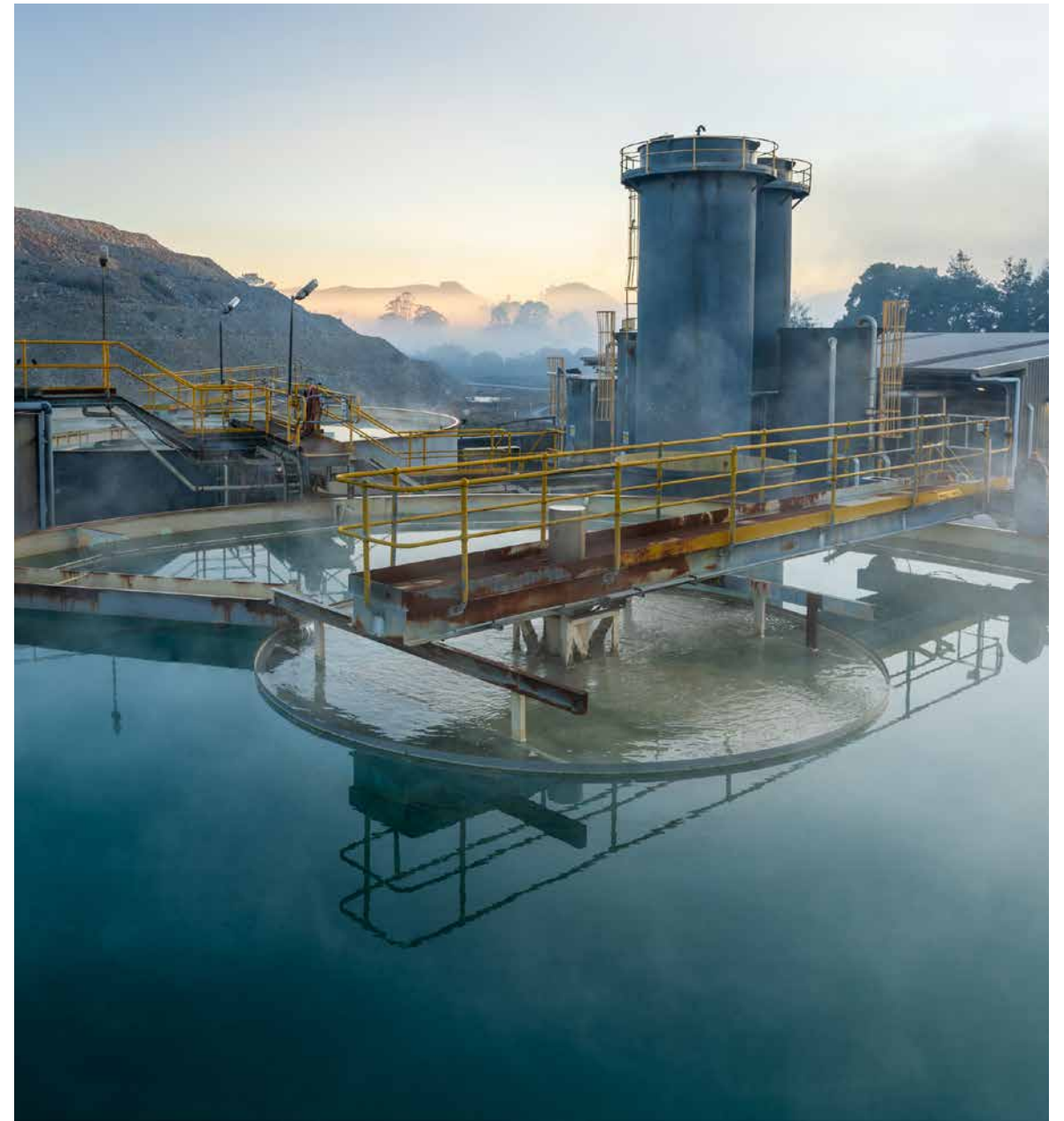
Water Treatment Plant at our Waihi Operation, New Zealand.
