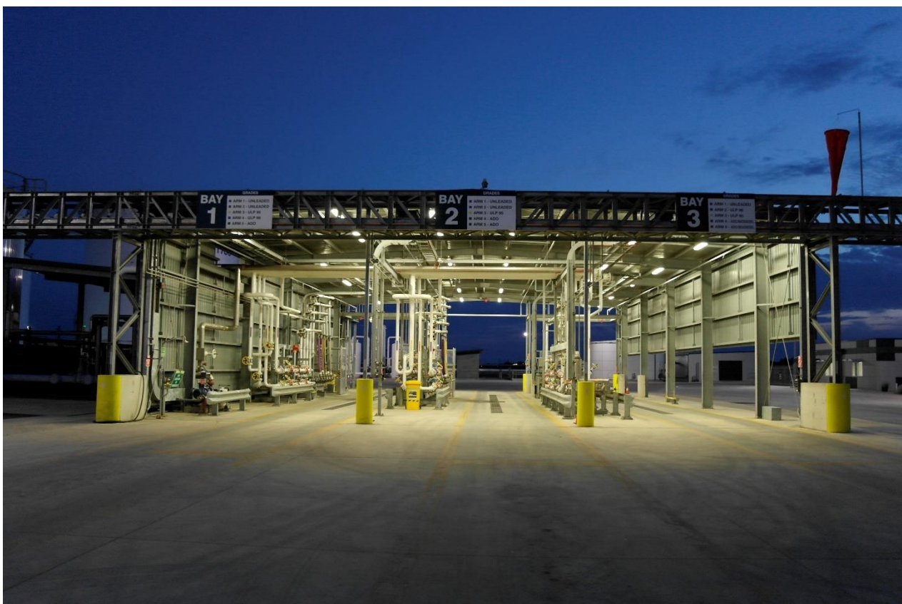
Above: Truck loading gantry at Pelican Point
